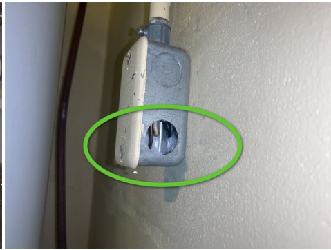
Missing knockout plate filler
